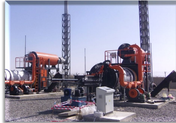
Municipal Waste Incineration System USACE Maywand Camp Site - Afghanistan
