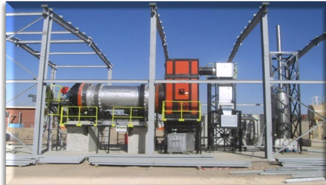
Sludge Incineration System – Kandahar Air Field NATO
